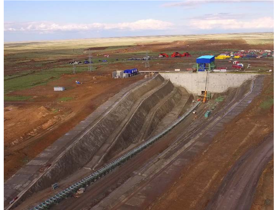
Primary crusher and conveyor
