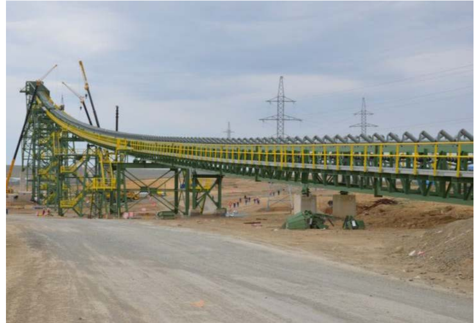
Conveyor – approach to stockpile area
