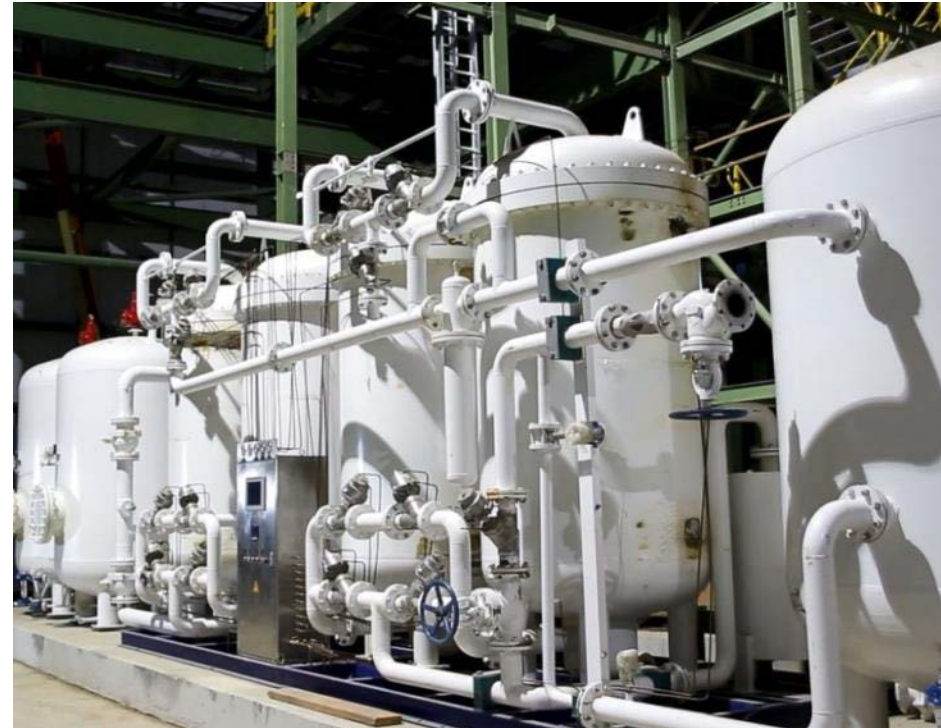
Concentrator water supply equipment
