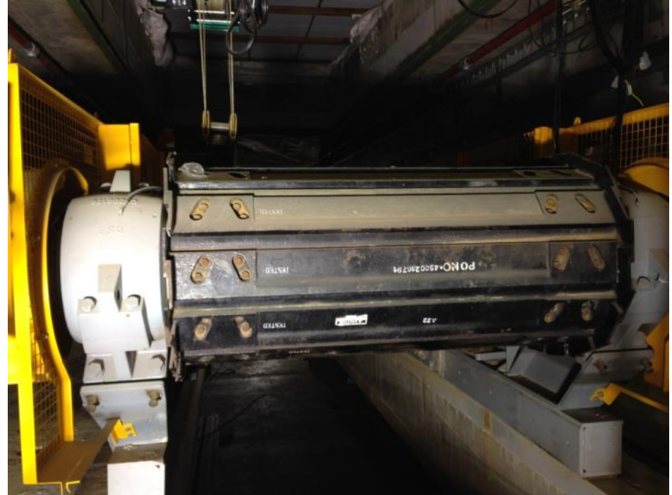
Ore stockpile reclaim conveyor
