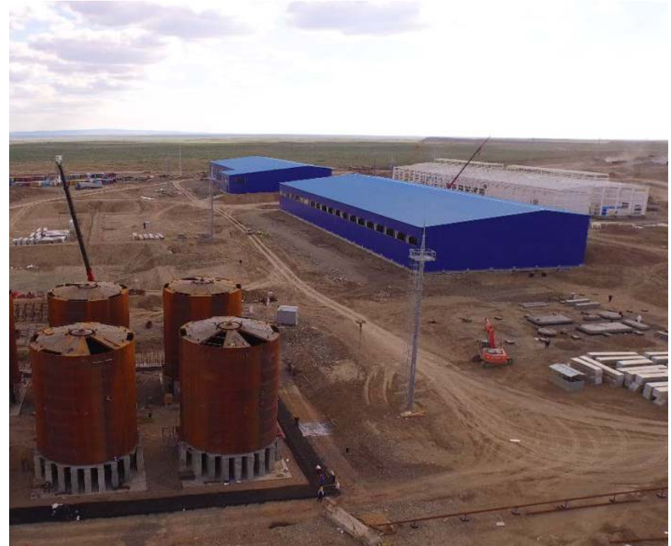
SX/EW processing buildings
