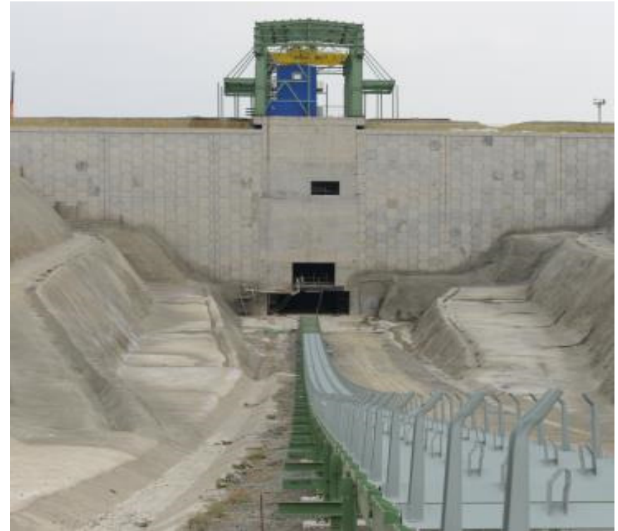
Primary crusher and conveyor
