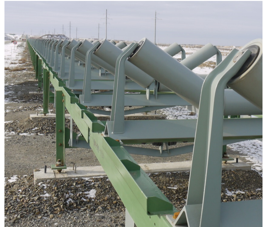
Conveyor - view towards concentrator facility
