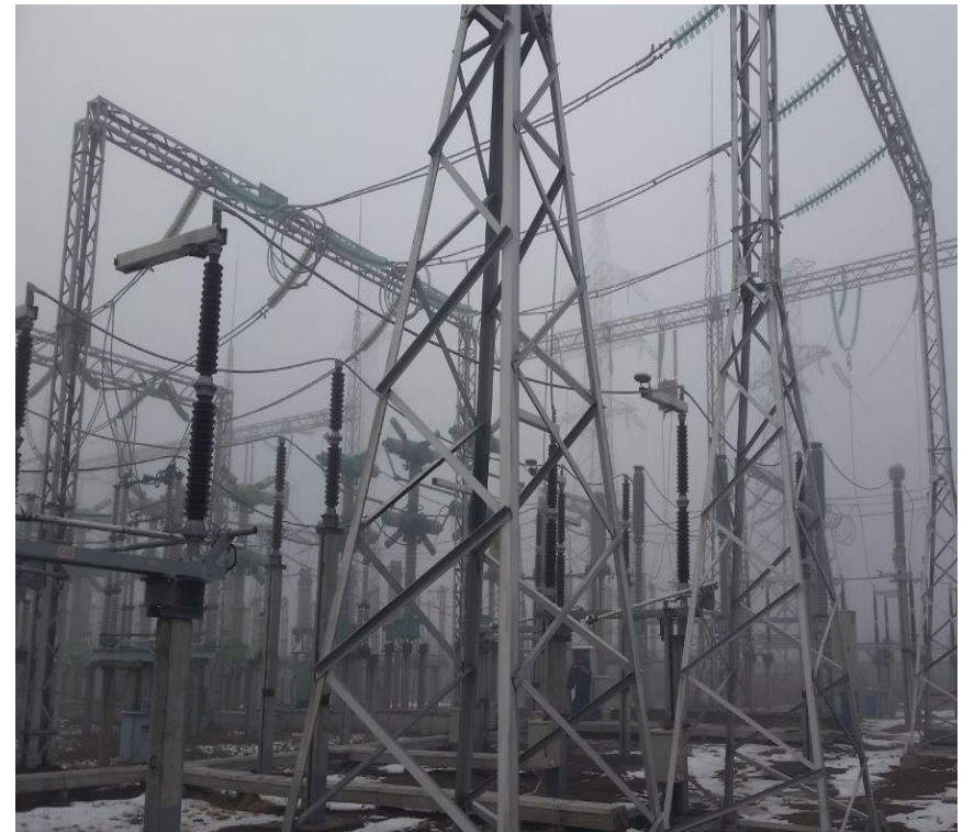
35 kv power lines
